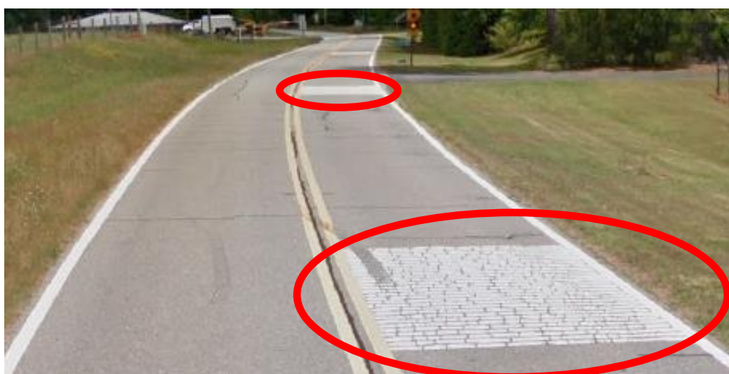
Figure 9. Transverse Rumble Strips
